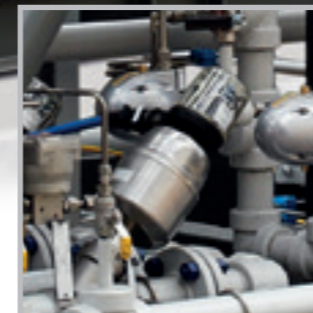
Process valves with limit switches
